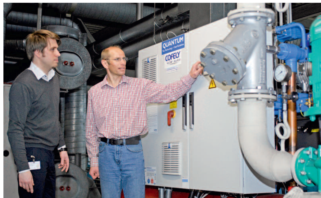
The Fogra energy efficiency expert, Maximilian Ondrusch (l.) and Werner Antretter, head of electronics/electricals at Süddeutscher Verlag Zeitungsdruck GmbH, standing in front of the new chiller.
