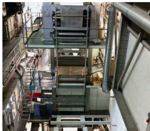
After the building of the steel base frame everything was ready in 2012 for the installation of the new press.
